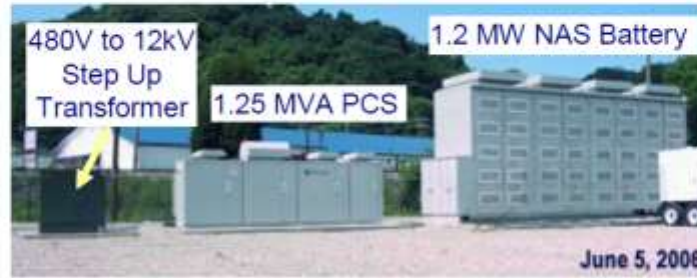
Figure 14 – Photographs of AEP's Chemical Substation before & after installation of 1.2 MW DESS in line with a 12kV feeder
